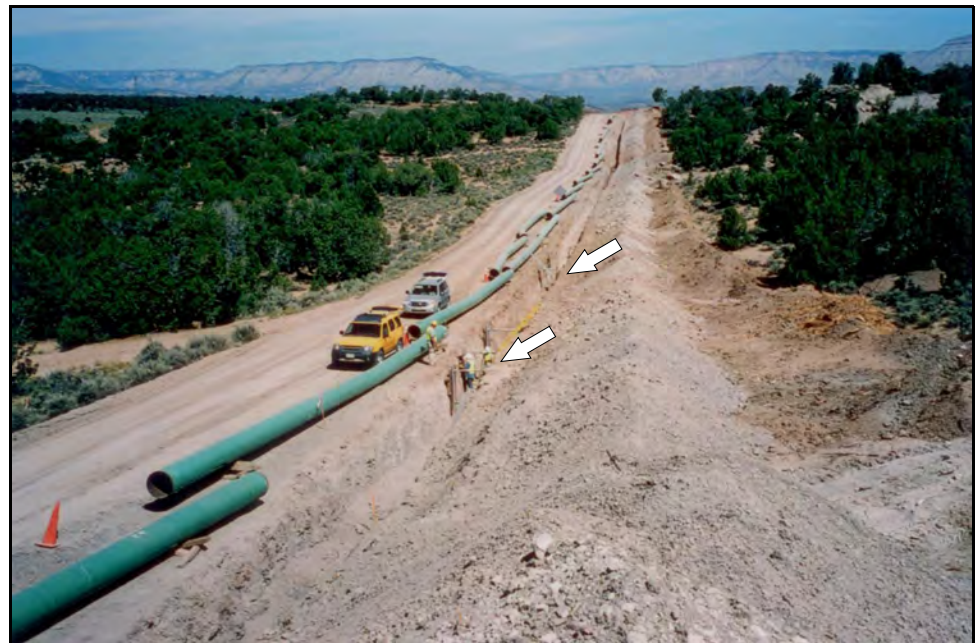
Plate 5.11-3. Photograph of trenching operations through site 5ME16789. Arrows indicate locations of the pit structures found along the trench walls.
